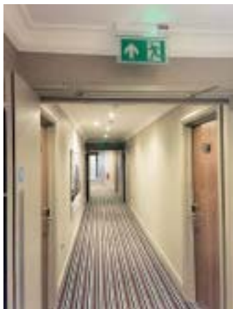
LED emergency exit signs have been used to create effective and comprehensive emergency escape routes throughout the premises.
